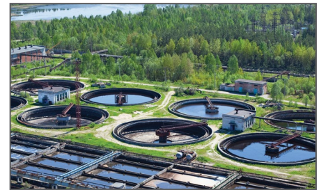
Water, wastewater treatment
